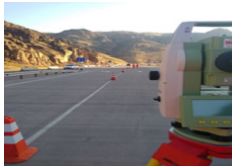
Figure 1. Measurements of the longitudinal profile of the cement concrete coating surface at the research site
